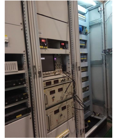
Power supply and control racks
