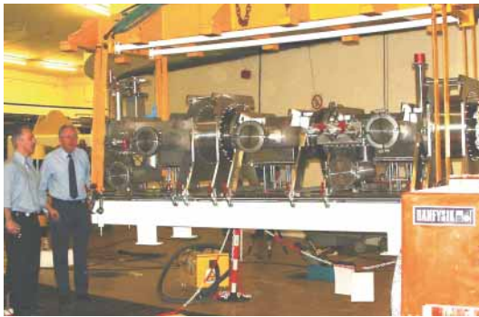
Fig. 4.6. Ian Gardner and Mike Krendler watch during the installation of new beam collectors and monitors in super period 1.
