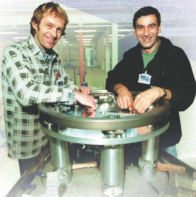
Preparations being made for the installation of the GEM radial collimator (01RC4033).
