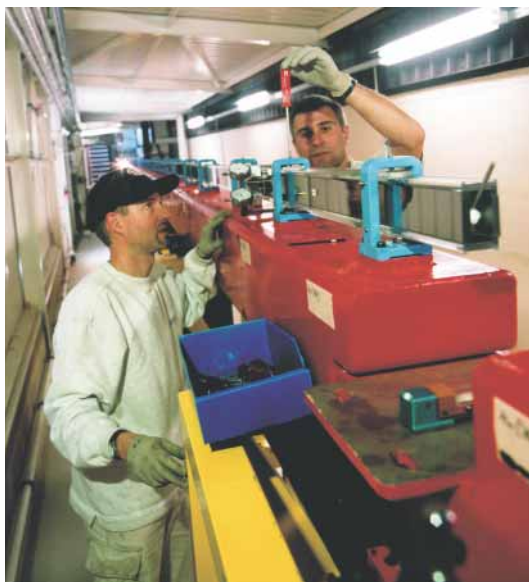
Fig. 3.5. Installation of the ENGIN-X guide by the team from Swiss Neutronics (02RC2110).
