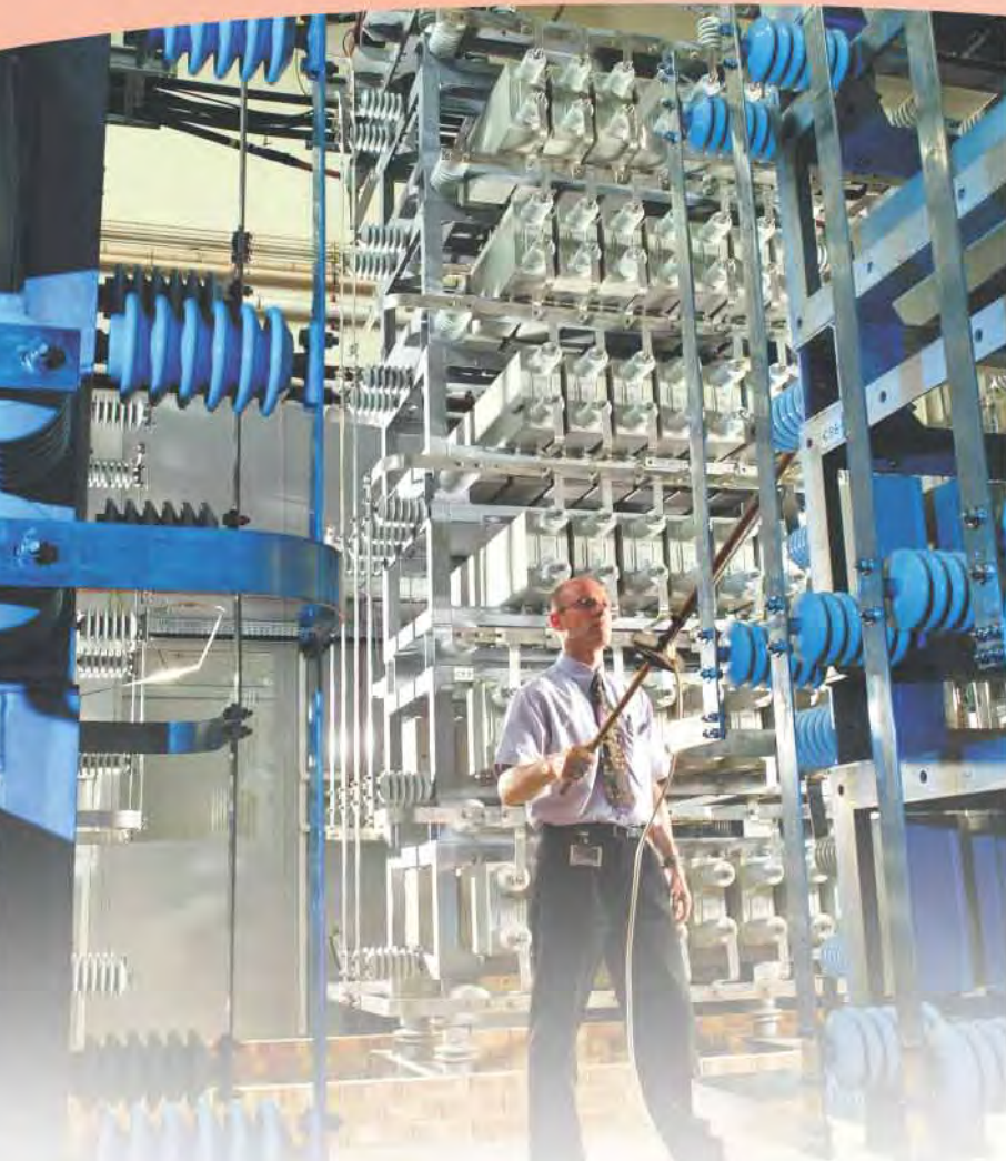
Fig. 4.5. Neil Meadowcroft inspects the new main magnet power supply capacitor bank (02EC3184).
